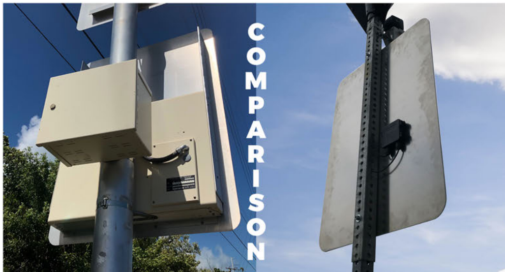
MOST COMMON LED SIGNAGE INSTALLATION
