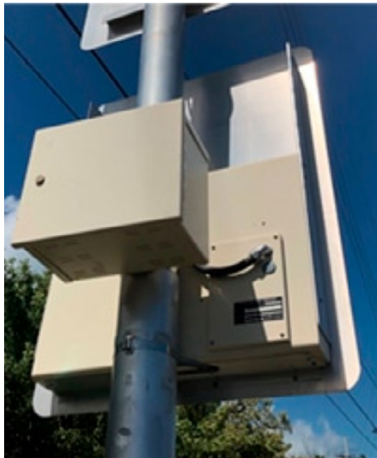
Most common LED Signage Installation
